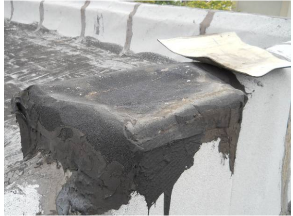
Poorly capped chimney between north building and middle building roofs
