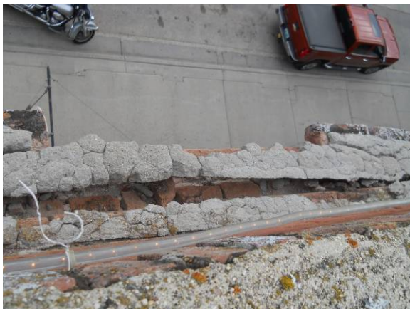
North building cornice: location where water had damaged grout and mortar of brick below, multiple bricks missing from ledge
