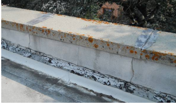
South roof: concrete coping with stucco on backside of parapet with visible cracking and metal flashing underneath
