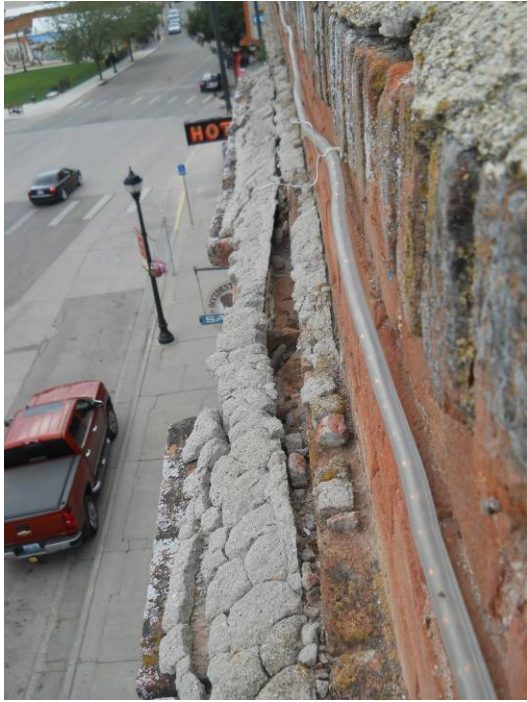
North building, deteriorating grout cap at brick cornices
