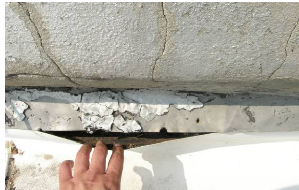
South roof: roofing membrane is not securely attached, existing metal flashing needs replaced, allows water and debris infiltration
