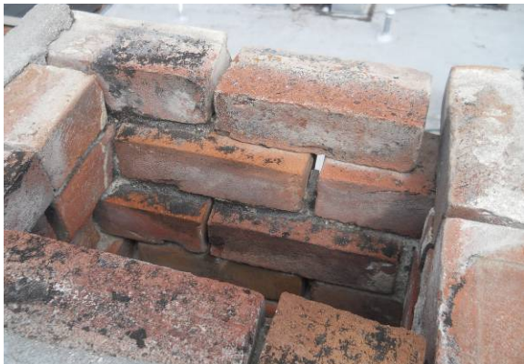
Typical chimney showing missing concrete cap, missing mortar joints, and loose bricks
