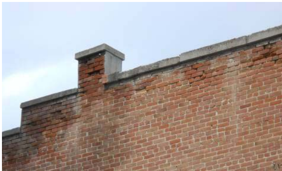
South facade showing deteriorated mortar joints and brick due to failing parapet joints, also showing water marks running down facade from joints
