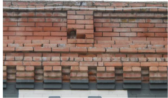
Upper portion of east facade, middle building showing eroded mortar joints and missing bricks
