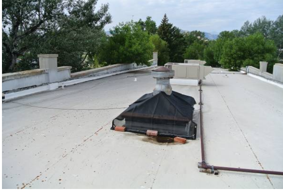
View of south roof looking west, showing existing single-ply membrane roofing material/condition
