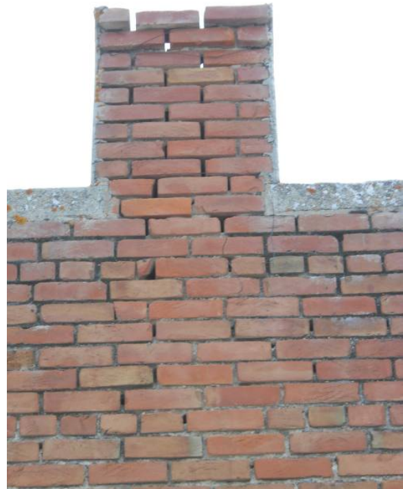
Chimney on north wall of south building showing fully eroded mortar joints exposing daylight
