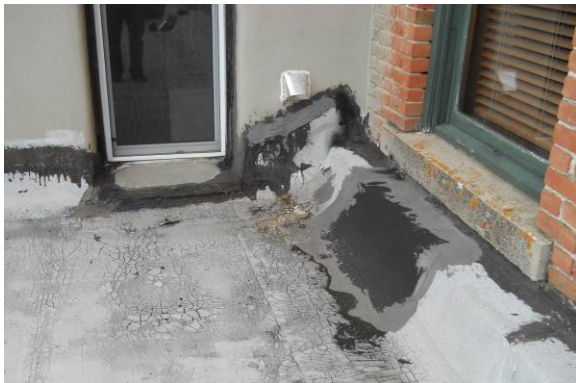
Typical condition of rolled roofing membrane, cracking/ hazing of surfaces, multiple patches, all providing water entry potential
