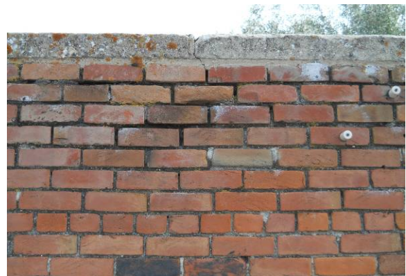
North facade of south building showing mortar joints eroded by failing joint in concrete parapet coping
