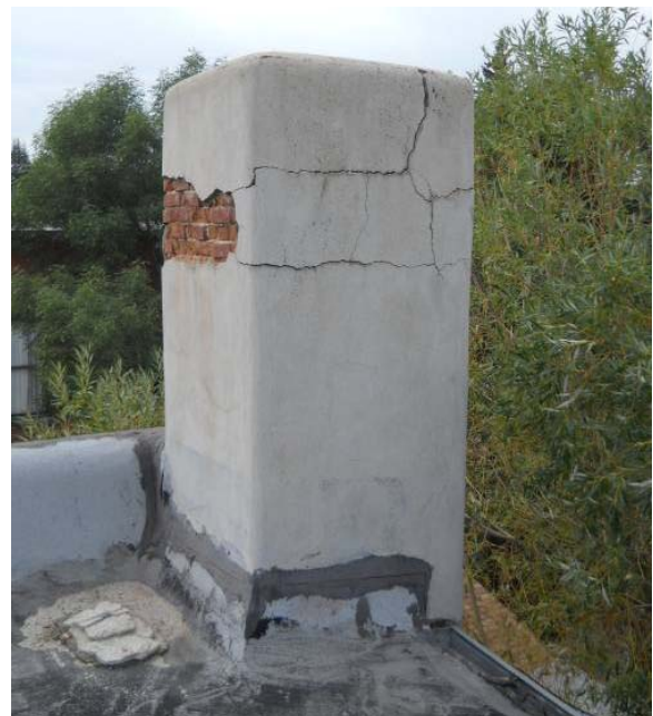
Chimney on southwest corner of north building showing signs of water infiltration through exposed inside and working its way through mortar joints and stucco to the outside
