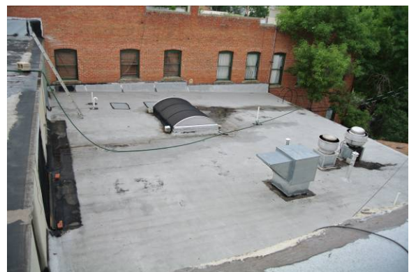
View of middle roof looking south, showing existing rolled roofing membrane material/condition
