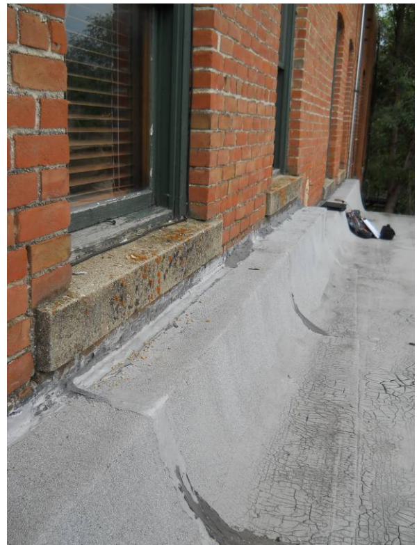
Curb at lower middle building roof to adjoining wall of south building
