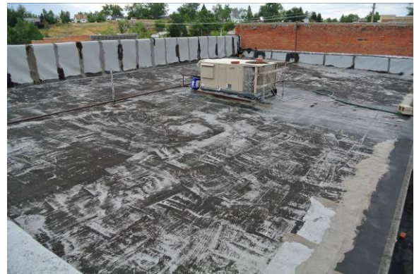
View of middle roof looking south, showing existing rolled roofing membrane material/condition with multiple patches
