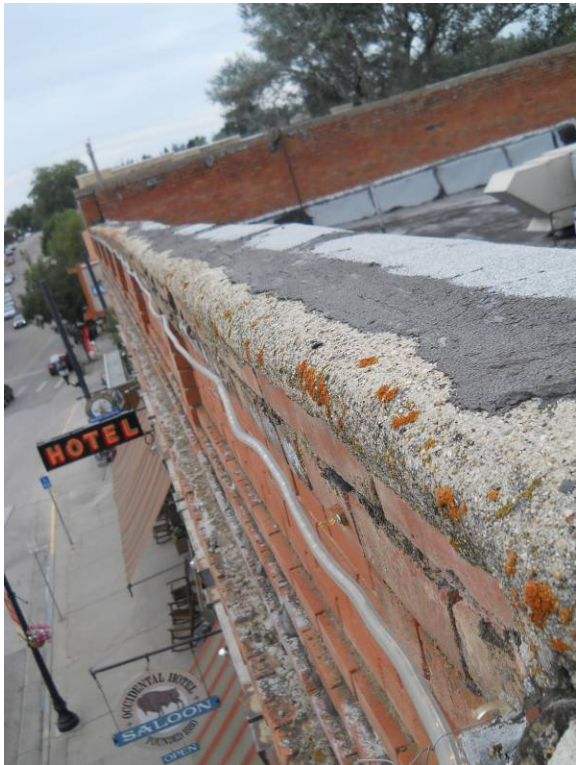
Middle roof: rolled roofing membrane terminating at top middle of parapet with concrete coping
