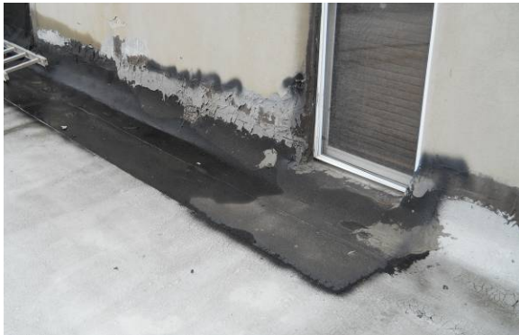
Middle roof: no continuous horizontal flashing, irregular existing caulk joint condition, multiple patches
