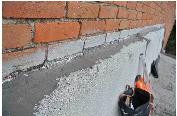
Upper middle building roof existing curb flashing at adjoining wall to south building
