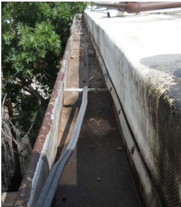
Gutter on south roof showing offset between top of roof and top of gutter (middle and north roofs are similar)
