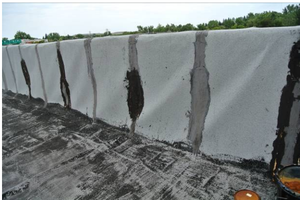
Roof material covering backside of parapet on east side of upper middle building roof
