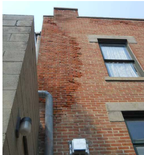
Large area of brick mortar erosion on southwest corner of south building
