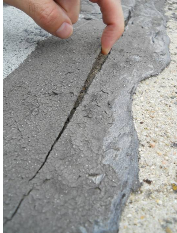
Cracks in rolled roofing membrane on top of middle roof parapet
