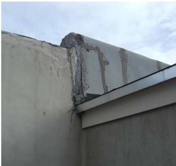
Middle to North roof: multiple patches, improper vertical flashing
