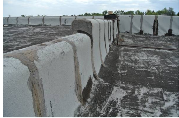
North and Middle roof: rolled roofing membrane over top of parapet wall with stucco finish underneath in most places
