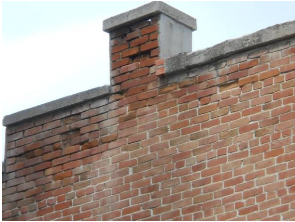
Typical brick and grout deterioration at south facade of south building
