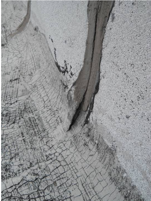
Typical cracking at seams in roof
