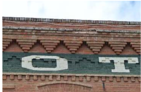
Upper portion of east facade, north building showing deteriorated mortar joints and brick
