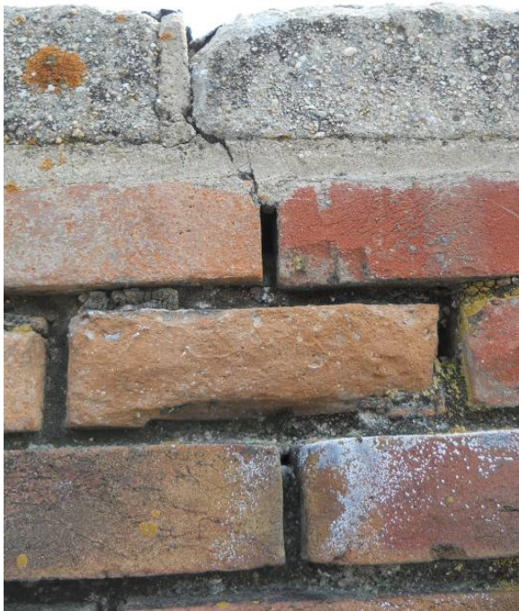
Front facade of south roof parapet showing path of water infiltration through the joint of concrete coping and eroding of brick mortar joints below
