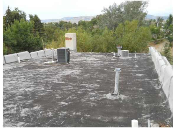
View of north roof looking west, showing existing rolled roofing membrane material
