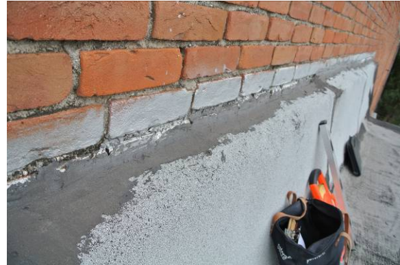
Middle roof: no continuous horizontal flashing against brick wall of south roof, irregular roof terminations provides opportunities for precipitation to infiltrate
