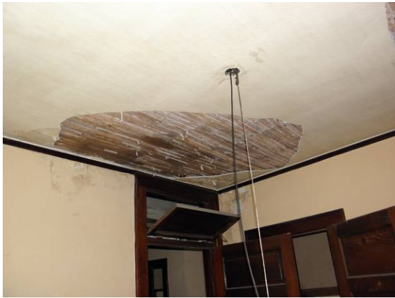
View of typical ceiling/wall water damage, missing plaster exposing wood lath substrate
