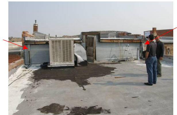
View of gutters and downspouts from upper roof discharging onto lower roof
