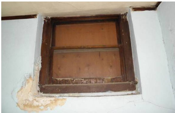
South window showing water damage
