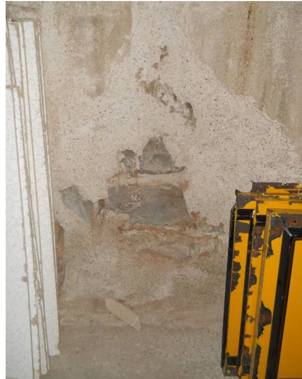
View of east basement stone wall showing sloughing material
