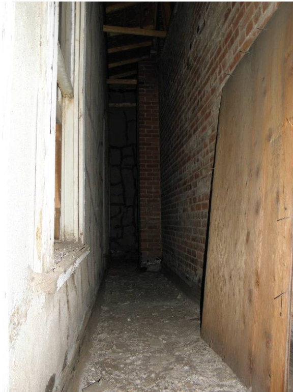
View from inside of covered light well on west side looking south
