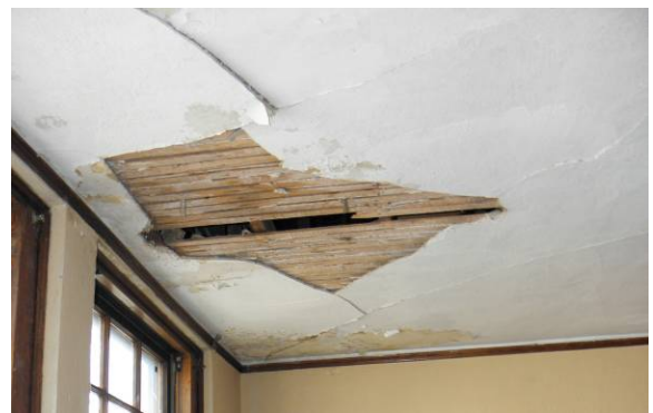
Typical ceiling damage from water infiltration
