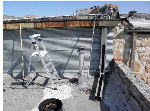
Gutter on east end of upper roof showing severity of offset between top of roof and top of gutter
