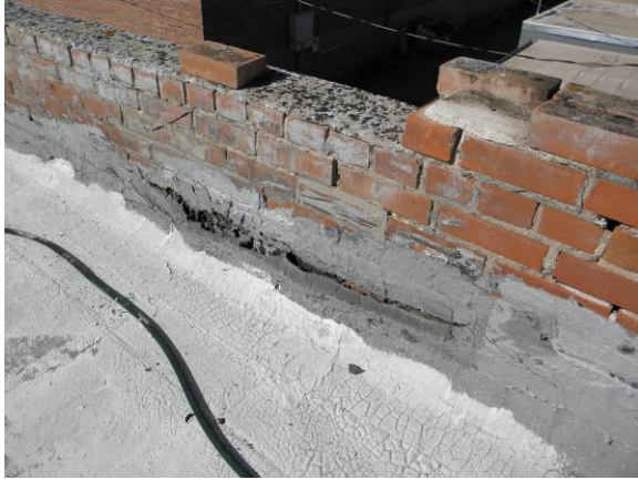
View of flashing at parapet where it is pulling away and allowing water/moisture infiltration
