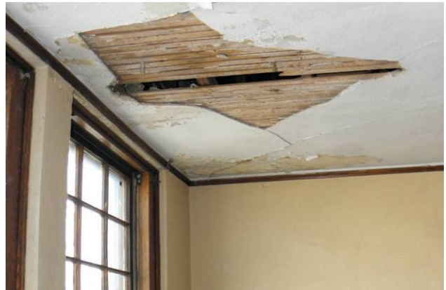
Ceiling damage in Room #1
