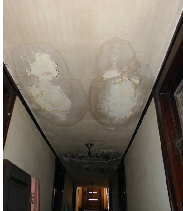
View of hall ceiling showing damage from water
