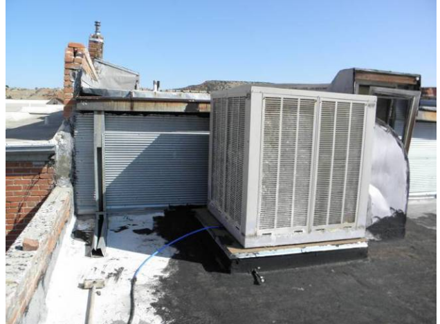
View of rooftop mechanical unit on lower roof
