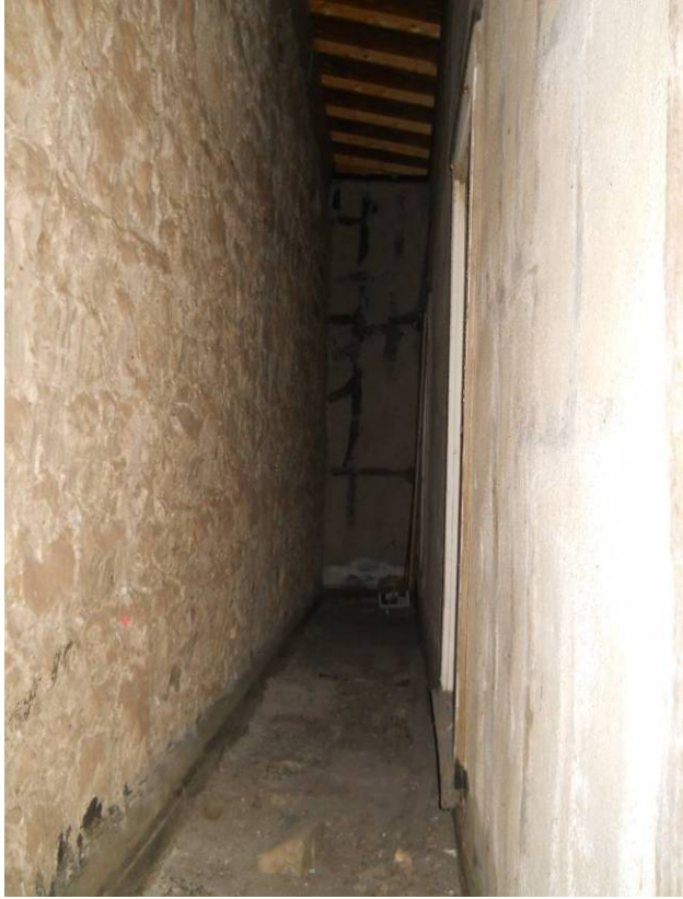
View of interior of east light well, looking south (west light well similar)
