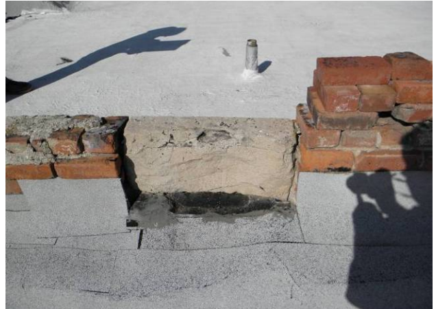
View of void in East parapet wall, looking West
