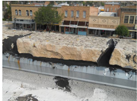
View of stone parapet cap from the rooftop showing joints not filled completely
