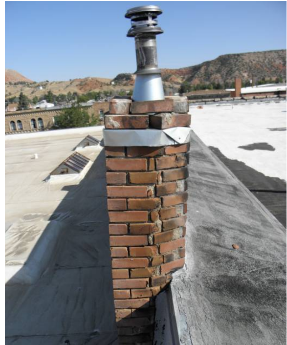
View of chimney with furnace vent - middle west side of the upper roof
