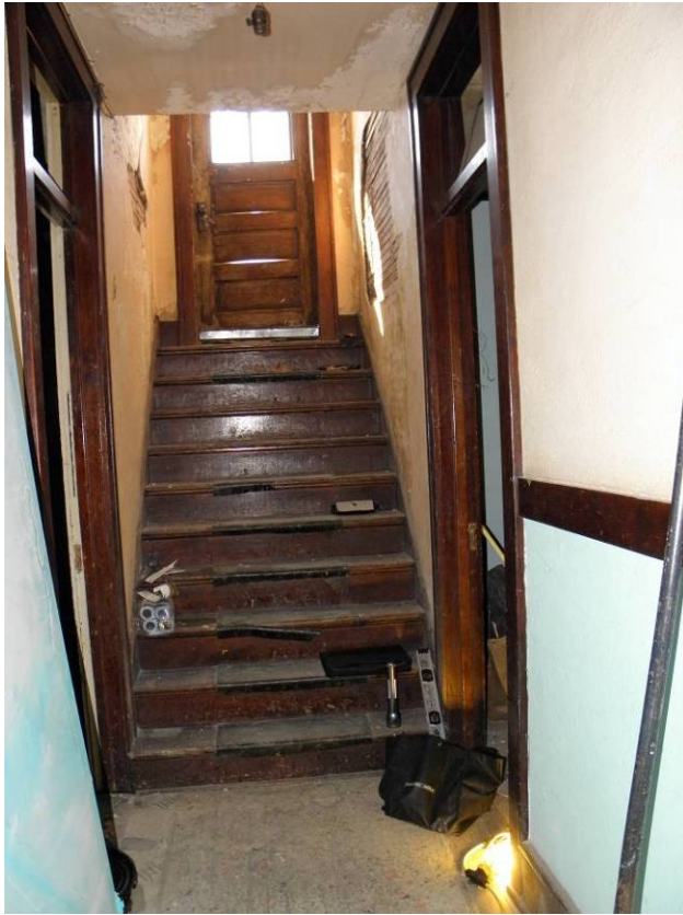
Stair and door to lower roof access at south end of main corridor
