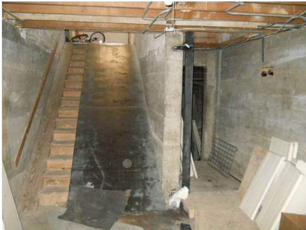
View of south stair and adjacent entry into boiler room
