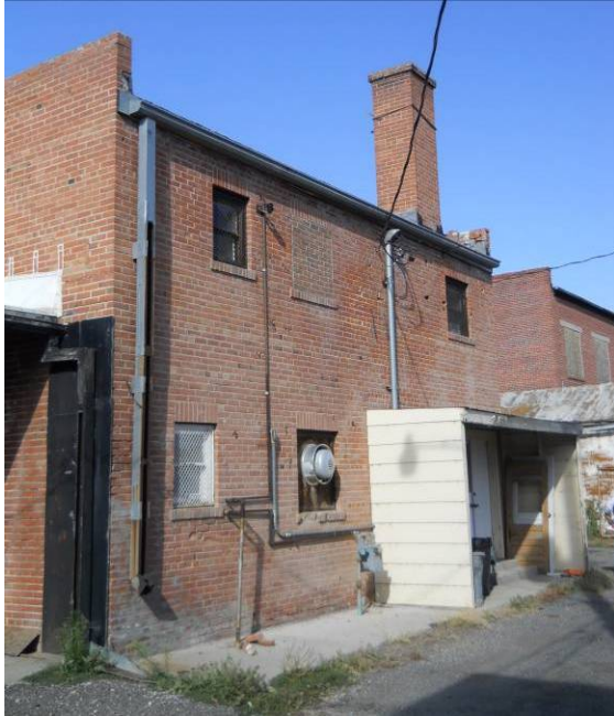
View of gutter and downspout from lower roof discharging to the ground/alley
